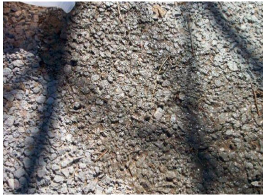
Figure 2.16: Clogged Pervious Concrete Pavement
