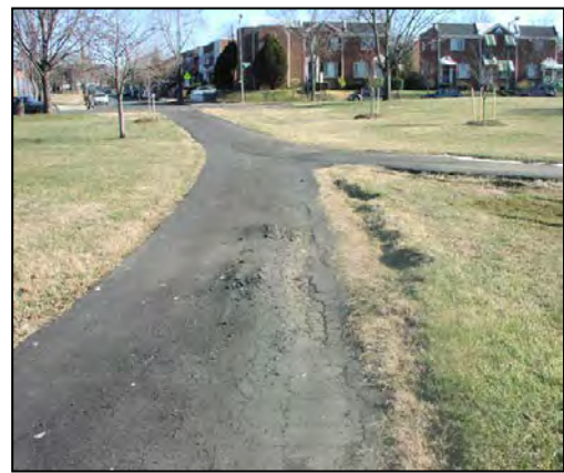
Figure 7.3 - Poorly Designed Trail Surface
