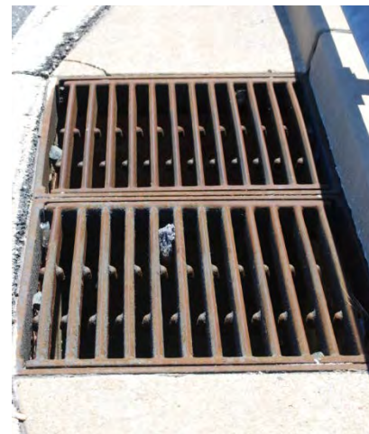
Figure 4.6 Non-Compliant Inlet Grate
