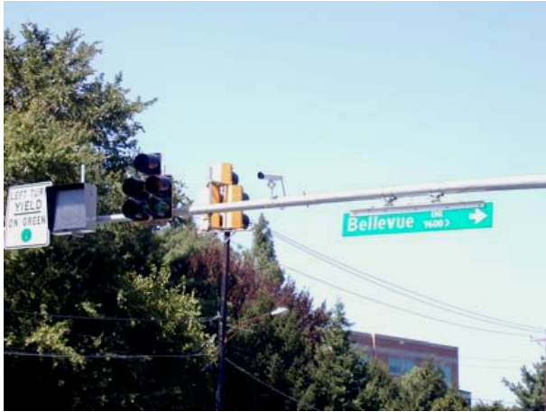
Figure 54 – Typical Video Detection Location (Mast Arm Mount)
