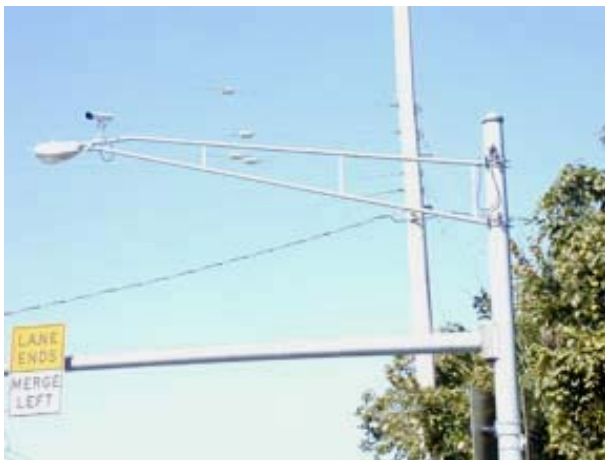
Figure 55 – Typical Video Detection Location (Lighting Arm Mount)
