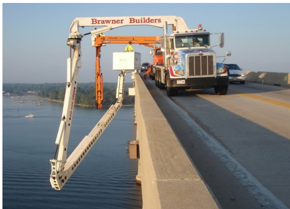
Figure 8. Under-Bridge Inspection Vehicle
