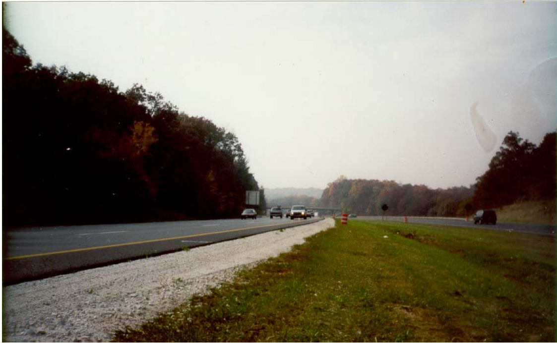
Photograph 1: Patches of grass visible in 6-week old gravel backfill on I-70
