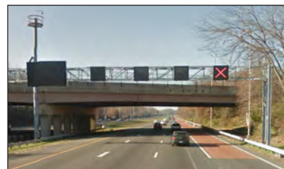
Figure 21: VSL Signs on Gantry on I-66, Virginia
