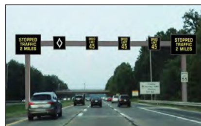
Figure 1: Advisory VSL Installation
