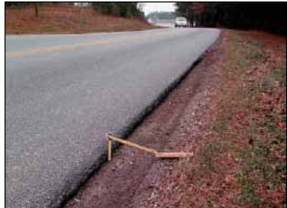
Figure 2.8 - Shoulder Drop Off Source: FHWA "Safety Edge" Brochure
