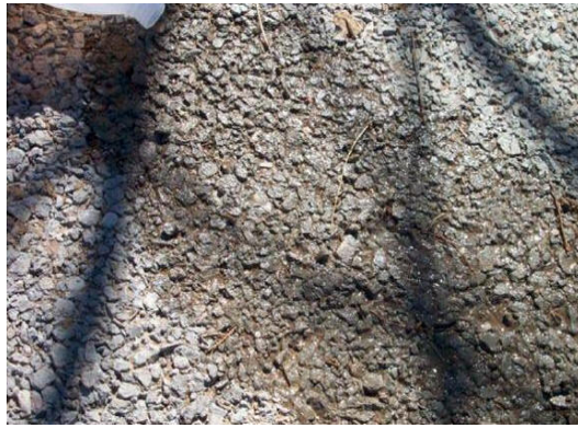
Figure 2.16: Clogged Pervious Concrete Pavement
